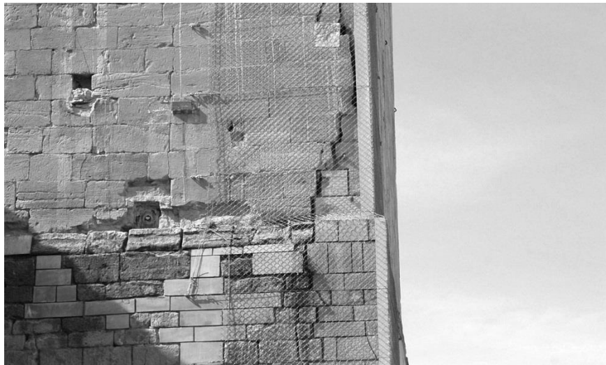
Figure 5: Tower of " Sta. Maria de Alcocer ": Damages caused by incompatible consolidation techniques manifest on matter in its appearance
